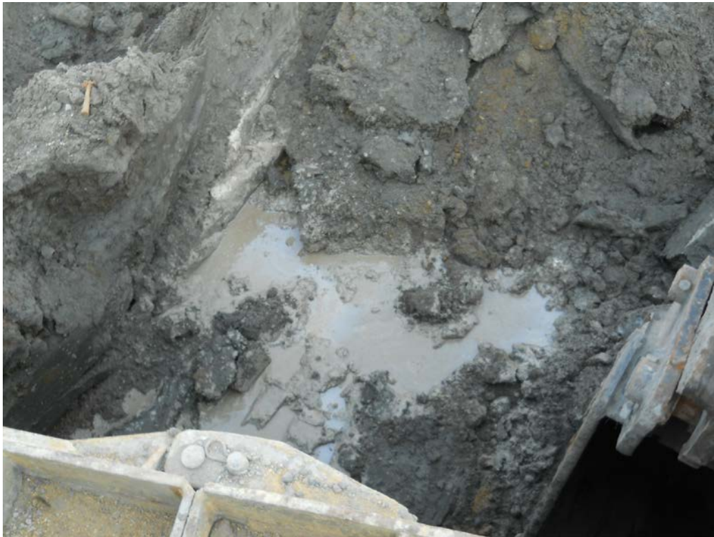
Visible sheen located in cell J3
