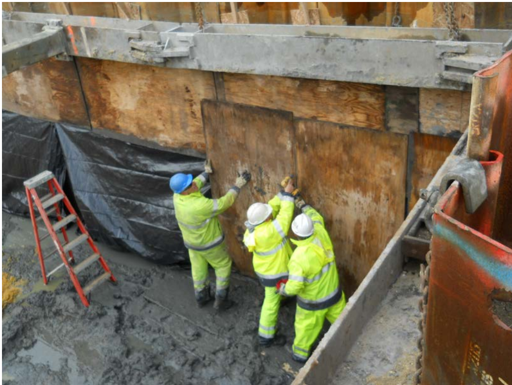
Installation of an impermeable barrier on the south side of the Remediation Area 1 excavation area
