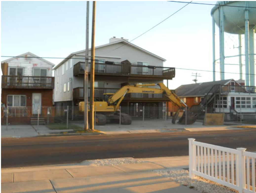
205, 207 and 209 40 th Street prior to demolition at the start of the Remediation Area 2 remedial action
