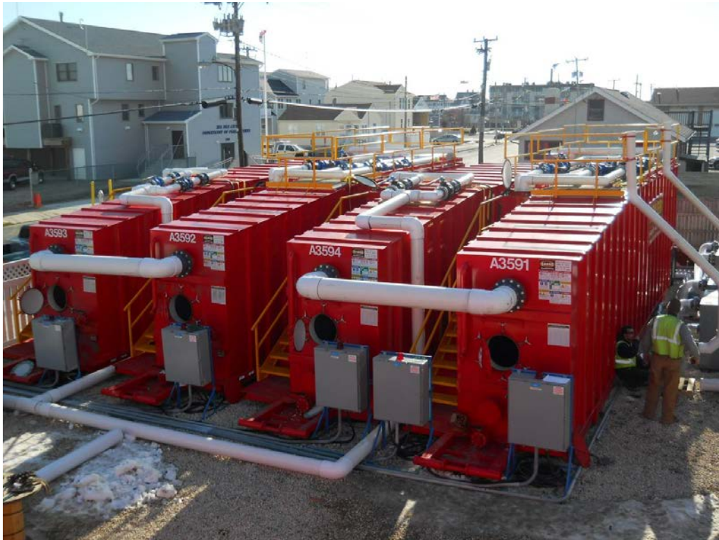
View of Depressurization System
