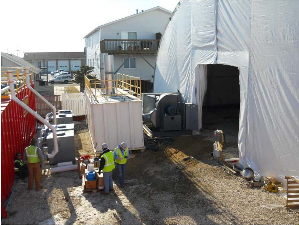
TIGG Air Handling Unit
