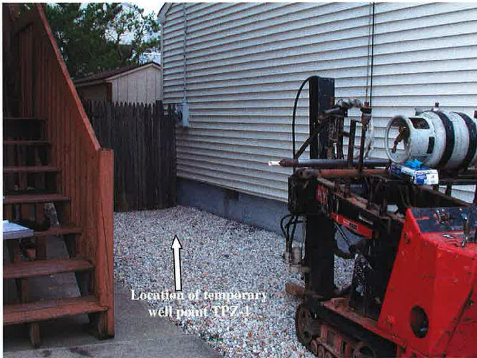
Photograph 2. 214 39 th Street: Vicinity of temporary well point TPZ-1 installed approximately 2.5 feet away from crawl space vent on the southeastern side of the residential structure.
