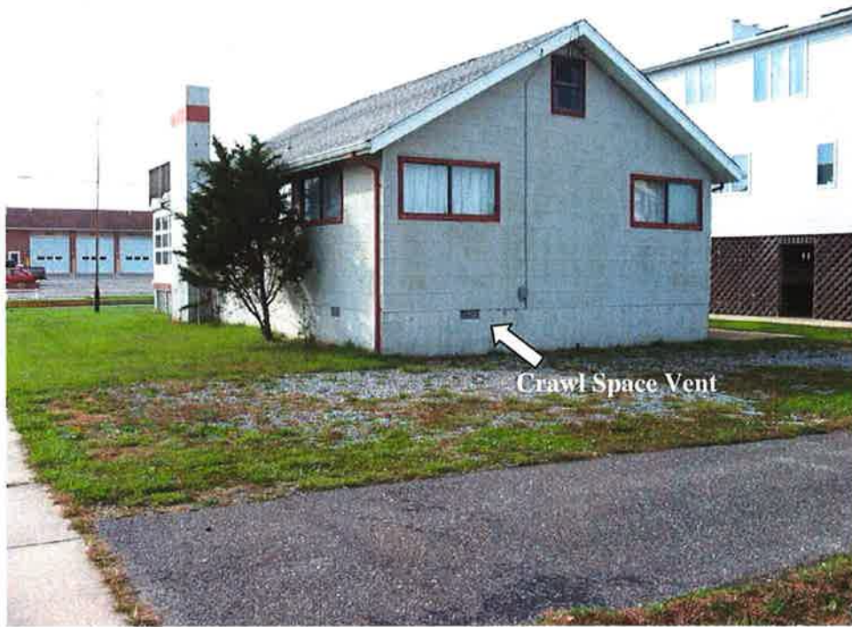
Photograph 3. 205 40 th Street: Crawl space vent on the northeastern side of the residential structure.
