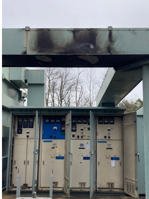
Figure 25: Monmouth Substation arcing event
