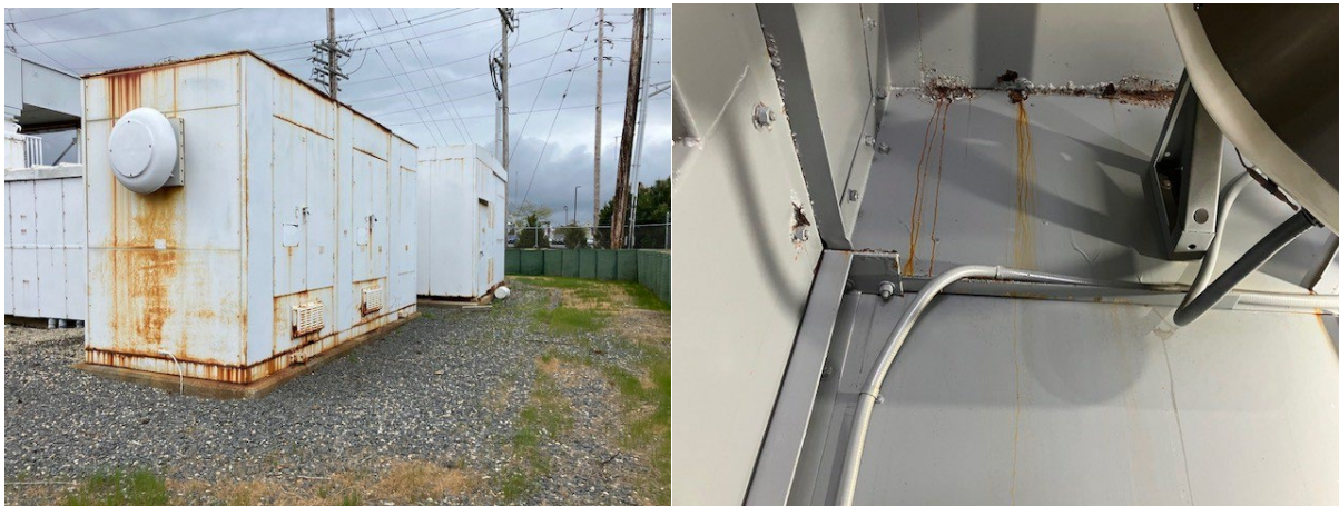
Figure 24: Ocean Beach Substation Switchgear
