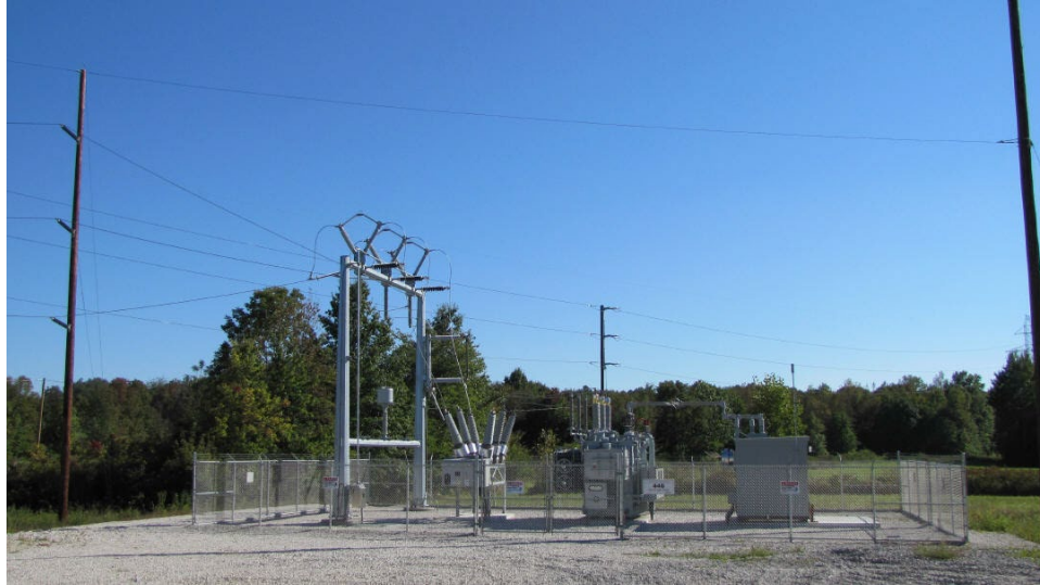
Figure 21: Typical Modular Substation
