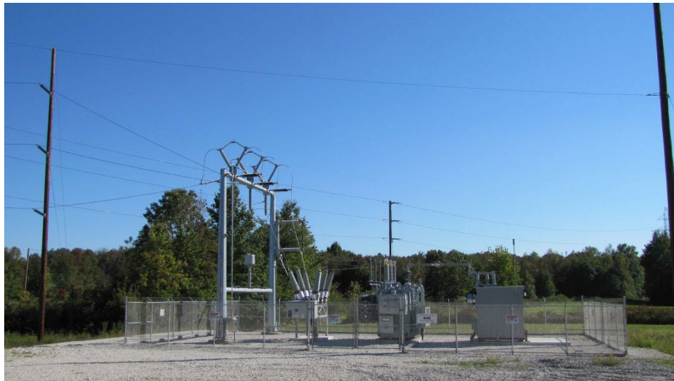
Figure 21: Typical Modular Substation
