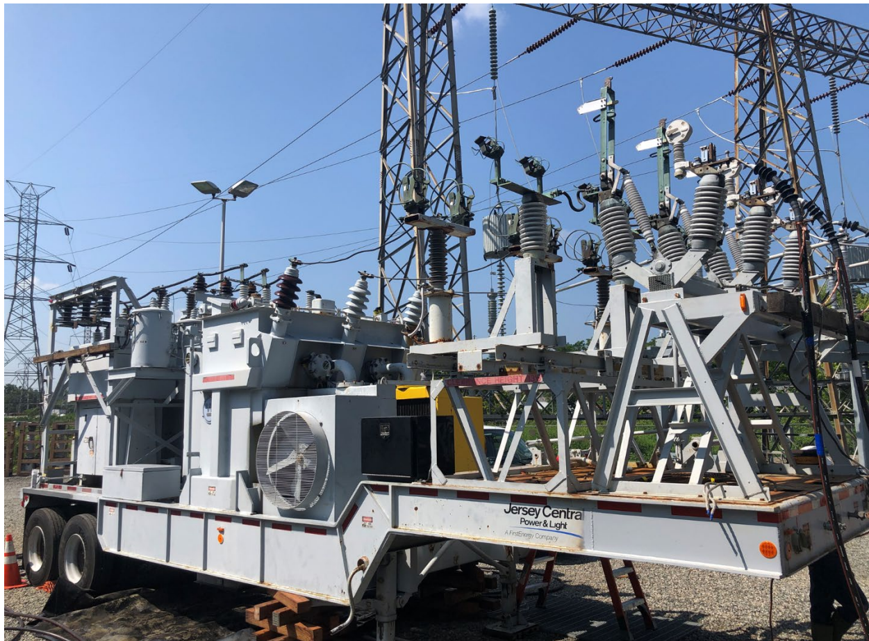
Figure 26: Recent Emergency Mobile Substation Installation
