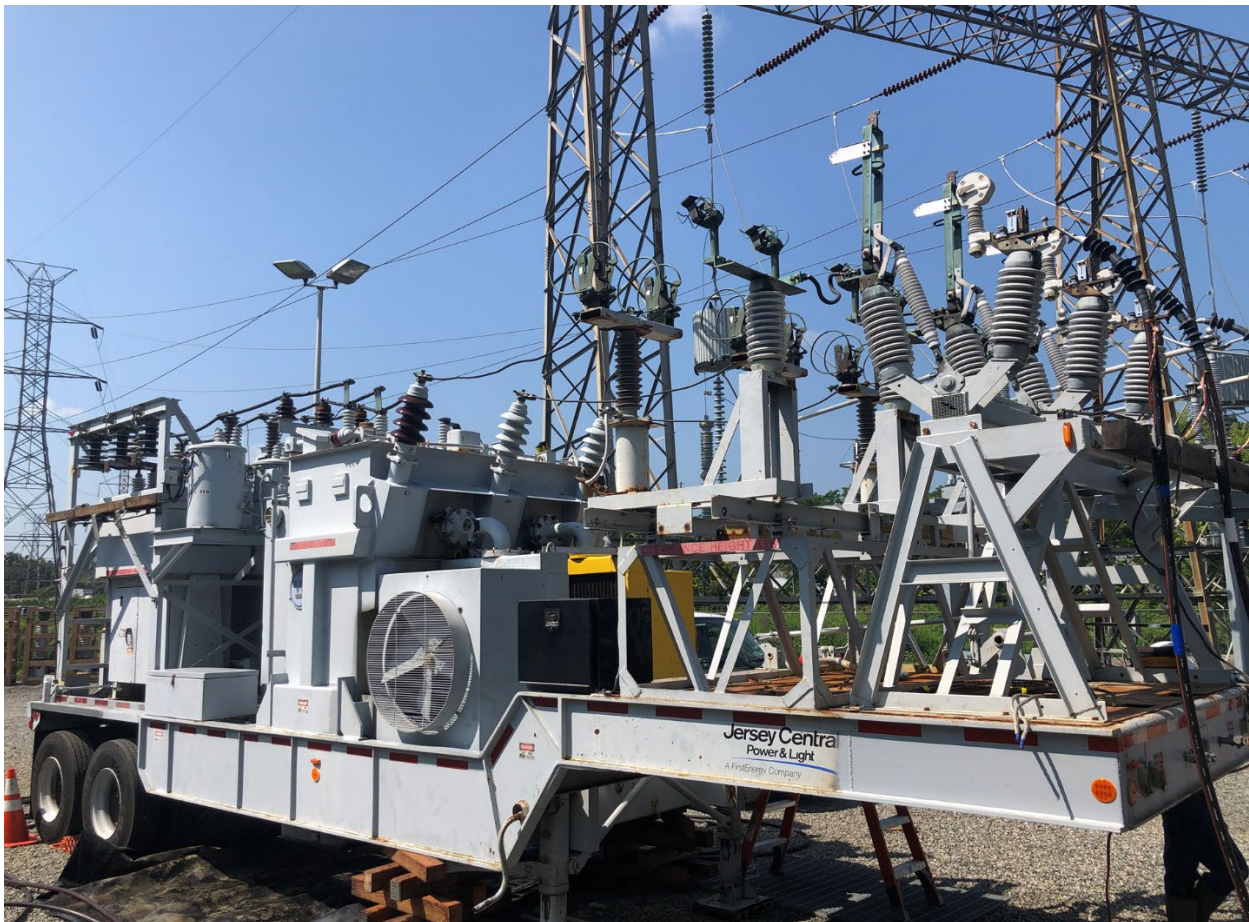
Figure 26: Recent Emergency Mobile Substation Installation
