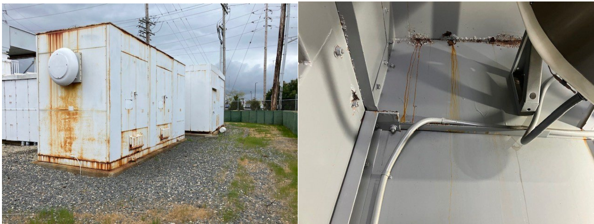
Figure 24: Ocean Beach Substation Switchgear
