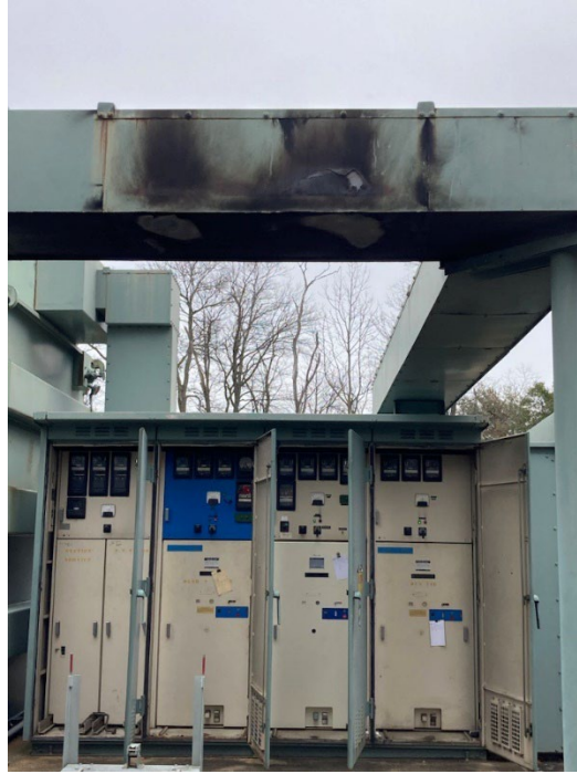
Figure 25: Monmouth Substation arcing event
