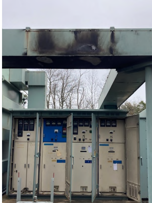
Figure 25: Monmouth Substation arcing event
