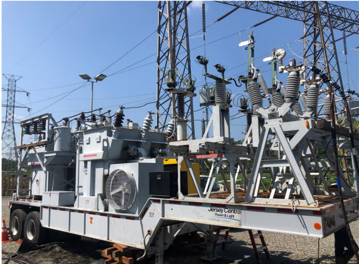
Figure 26: Recent Emergency Mobile Substation Installation
