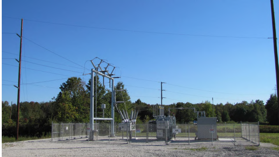
Figure 21: Typical Modular Substation
