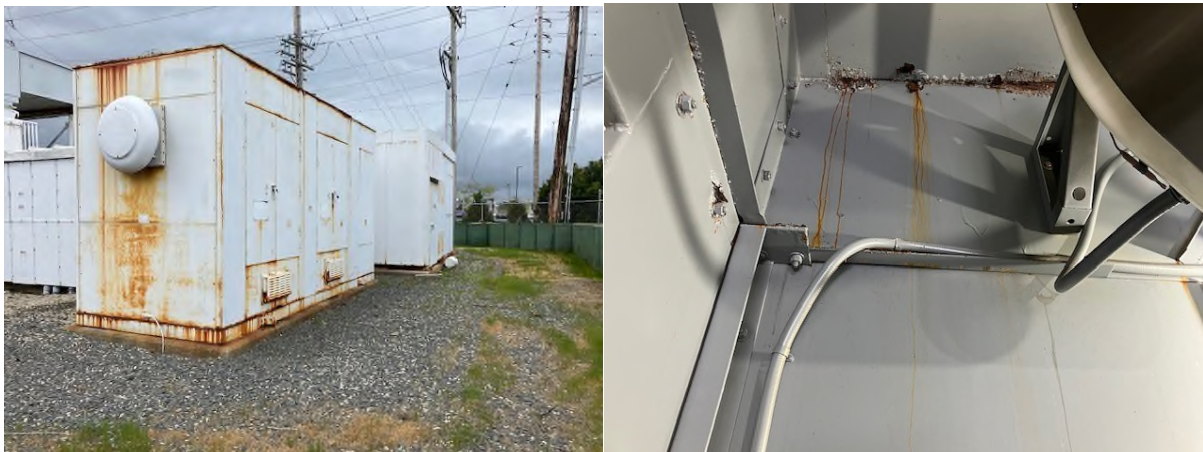
Figure 24: Ocean Beach Substation Switchgear
